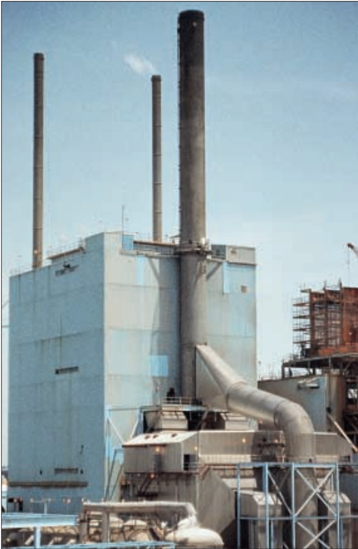
Pulp and paper recovery boiler
