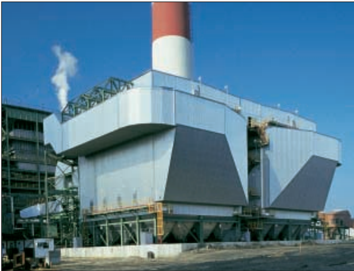
Precipitator with 16-inch wide plate spacing on a 320-megawatt coal-fired power boiler
