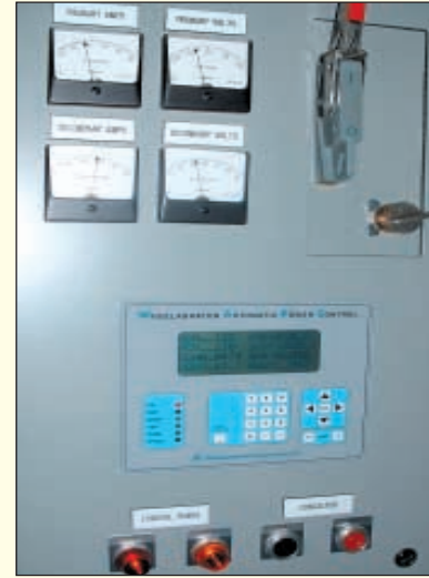
Automatic Power Control
