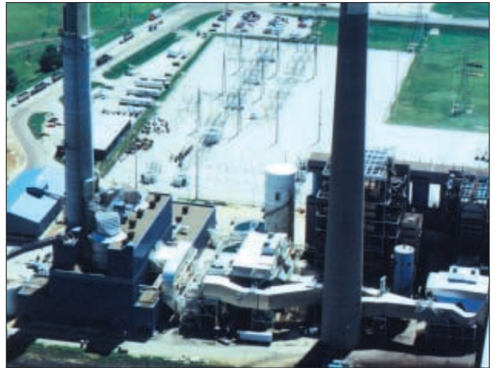
Precipitator and Wet FGD System controls emissions from two coal-fired boilers producing 440 megawatts of power
