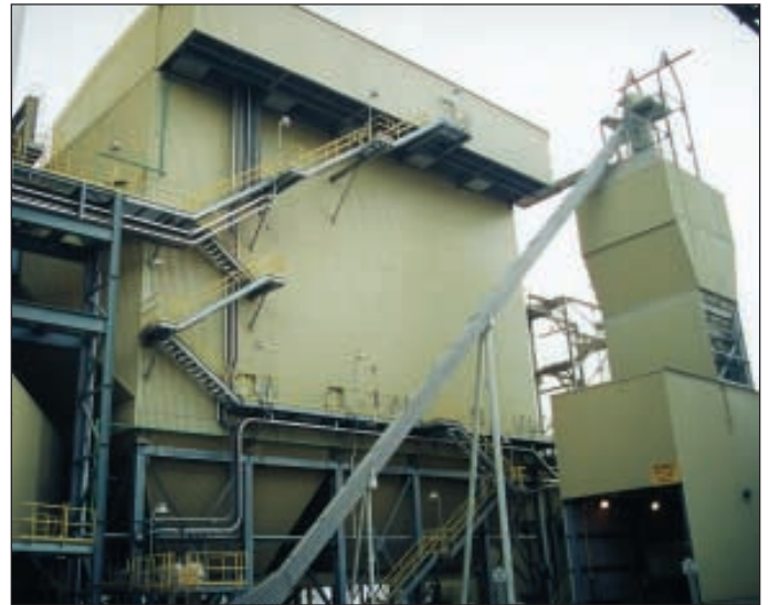
Pulp and paper power boiler
